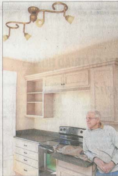
The renovation of the Queen Anne home moved to 408 Cedar St. last fall was recently completed by contractor Southern Evergreen. The project was part of an effort to save the house, moved from Blandwood Avenue in September. Preservation Greensboro Inc. and its supporters orchestrated the relocation when plans for a new jail threatened the structure, which preservationists estimate was built in the early 1900s.
