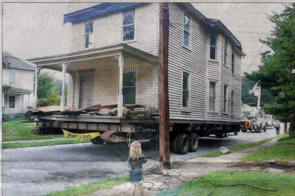
Jackson Prause waits as the house is slowly prepared to be moved down Cedar Street last month. The jobs of moving telephone, cable and power lines, as well as the house itself, required dozens of professionals for the Sept. 19 effort. The project to preserve the home was started by the Zenke family, who have received help from individuals, companies and organizations, including Preservation Greensboro, Southern Evergreen and the city of Greensboro.
